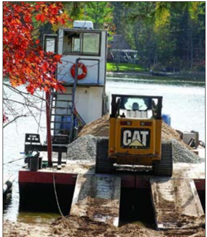
When working on islands or boat only access land, everything needs to be shipped in, including good fill like this load of sand and gravel. Anderson Barging Captain, Casey Sundahl operates the company's CAT 287C multiterrain loader to offload the product.
